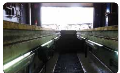
Example of LINE LIGHT solution mounted in a truck mechanic's pit
