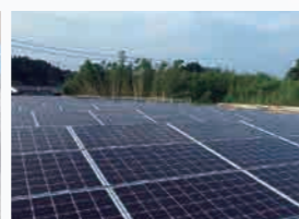
Kagoshima Solar Power Plant
