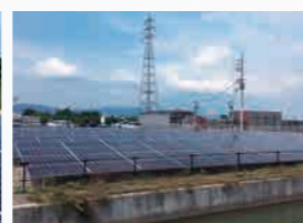
Wakayama Solar Power Plant
